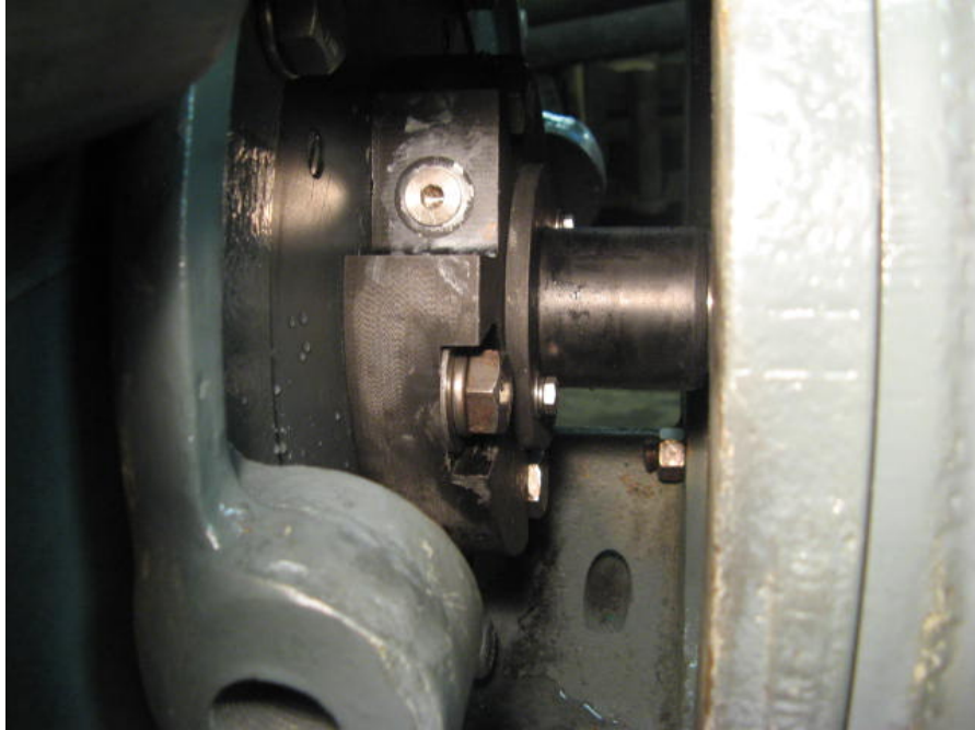
Post-Blow #6 Pump to Motor Packing Seal Ring Figure 2
